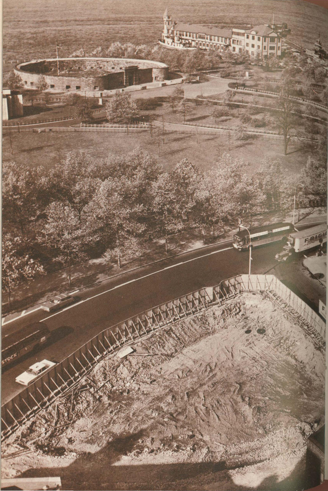
View of Battery Park, including historic landmarks, from where new building to be located. Foreground area shows building plot being excavated.
