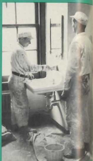
NEW FACE — Workmen applied spackle to the 300th hotel room last month preparatory to painting. SCI's rotating maintenance plan calls for redecorating 650 rooms periodically. The 115 rooms on the 9th floor were completely modernized in 1959. The maintenance project which includes re-surfacing of walls, painting of furniture and floors, requires 1,000 gallons of paint per year. Many appreciative seamen have commented on this upkeep program.
