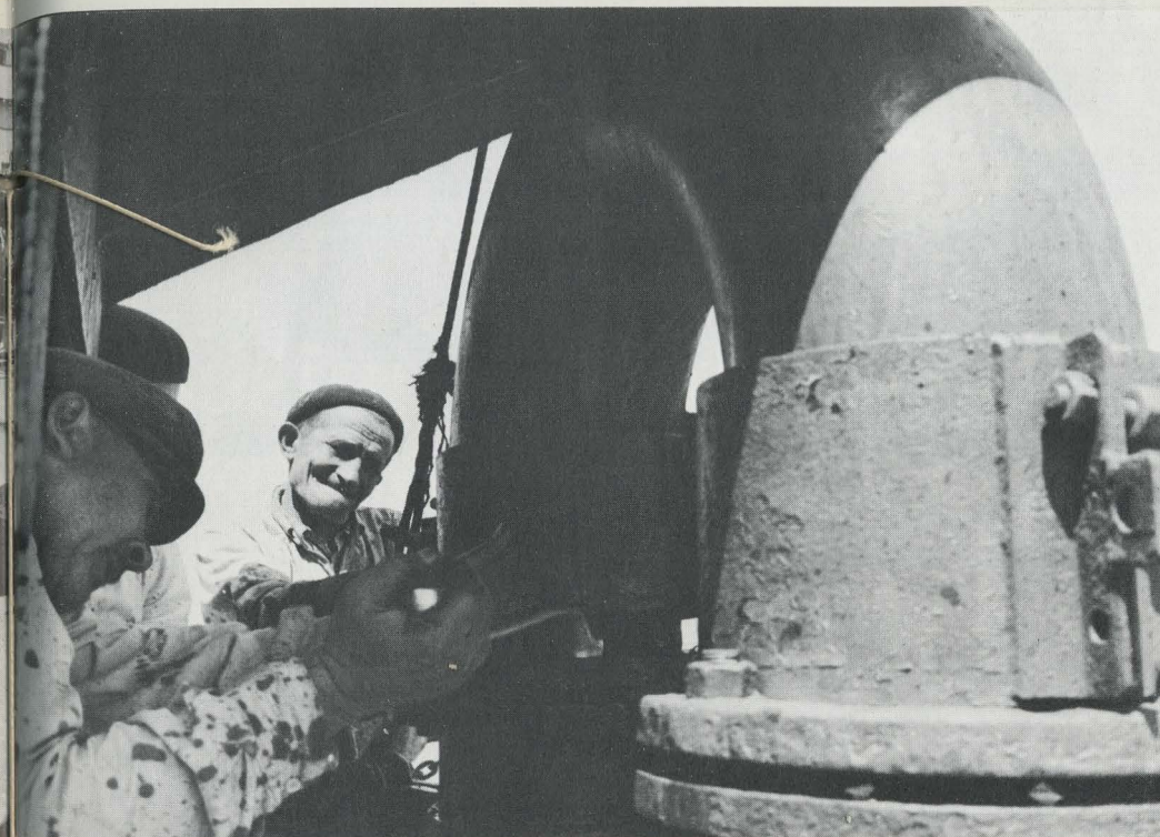
A faulty connection in the piping system could mean disaster at sea—as these men who are experts at their work know too well.
